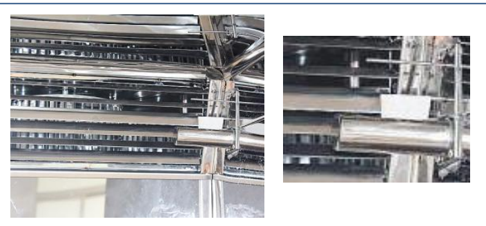
Temperature and Humidity Sensor
